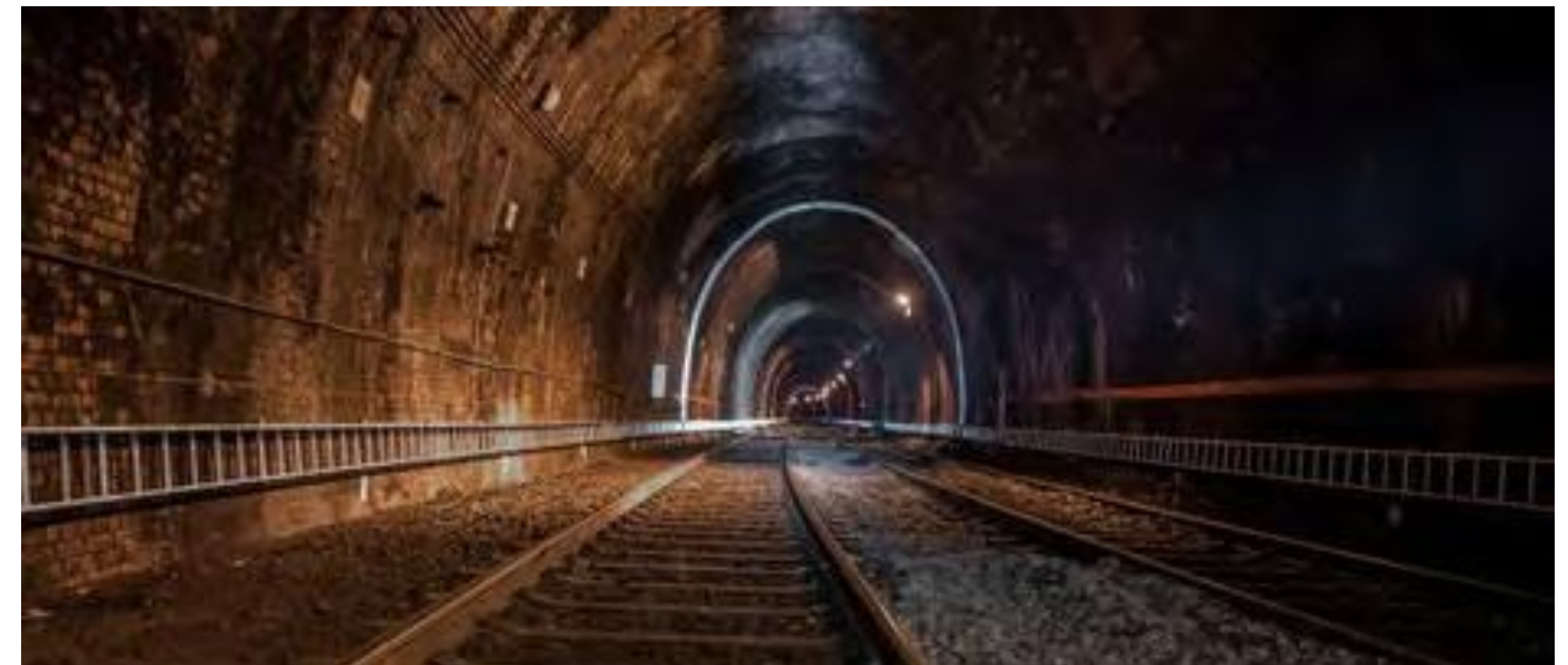
Including Electrification of Phoenix Park Tunnel along with installation of Slab Track
